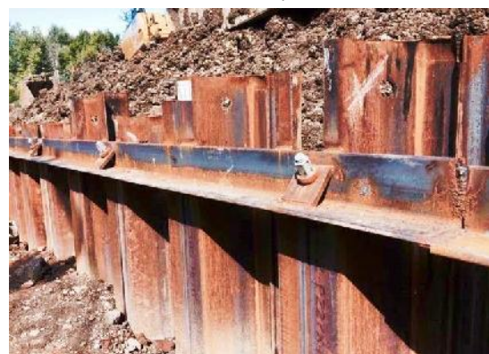
This is a view of the finished sheet piling wall used to stabilize the embankment.
