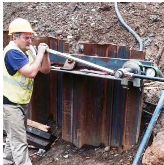
A worker applies tension to the tieback anchor at the top of the sheet pile.
