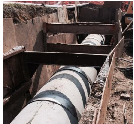
This is a view of the pipeline before backfilling. Notice the 12 inch wide stainless steel straps.
