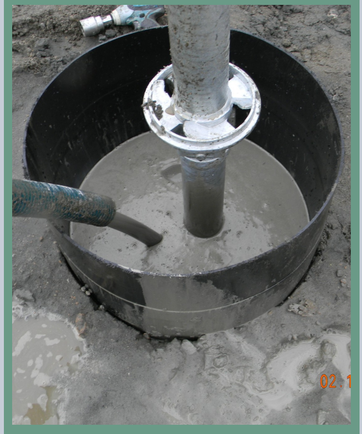
Typical MVP Installation
