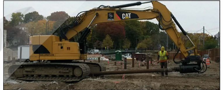
The 8.625" diameter by .408" wall with 18" and 22" helix bearing plates were installed in 20 ft. and 25 ft. sections using a 80,000 ft. lb. torque motor. All sections were bolted together.
