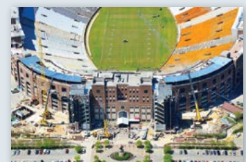
Construction underway on south end of stadium (Image courtesy of Aero Photo)
