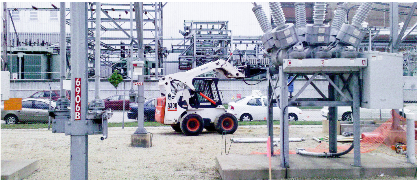
Installation below 69,000 volts
