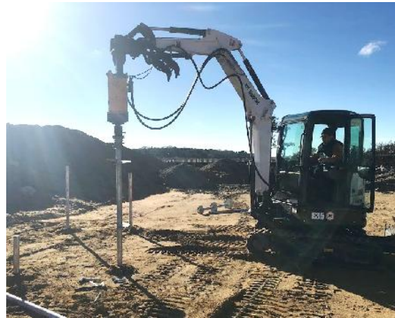
This photo shows a track machine installing an ECP Torque Anchor™ on the job site.
