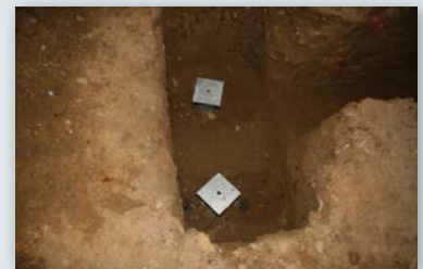
Battered piles installed within saddle beam excavation and fitted with new construction brackets
