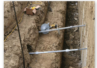
Leads and extensions with helix plates set in place on south side of wall
