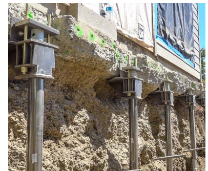
Underpinning piers and grouted tiebacks in place after first stage of excavation
