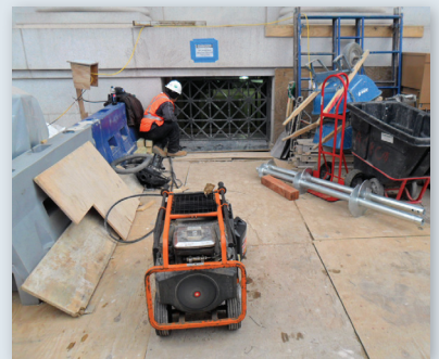
Remote hydraulic source located outside the building
