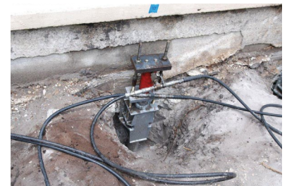
Hydraulic cylinders connected to brackets
