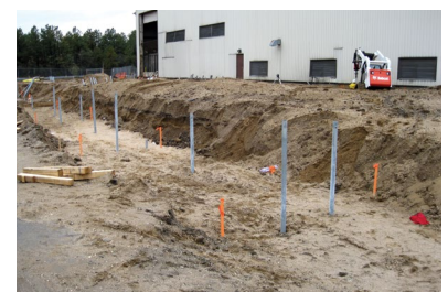
Helical piles installed along grid line ready to cut to design elevation
