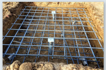
Installed piles fitted with new construction brackets to be cast within reinforced pile cap
