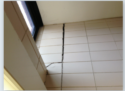
Cracks observed in CMU partition walls
