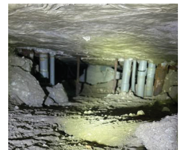
Void under electrical room prior to PolyLevel injection
