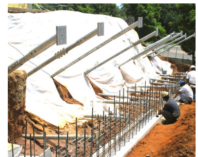
Helical tiebacks completed and ready to be cast into new concrete retaining wall
