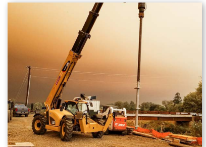
Telehandler with 20 feet of drive tooling and 7-foot helical pile lead section
